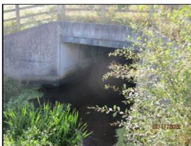
Photo 3.5.2 Showing the culvert area where there are silt deposits suitable for lamprey
